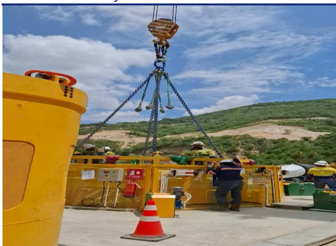
Exhibit 7. BRMS underground mine air flow installation
